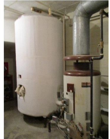
Photo: Main Water Heaters
