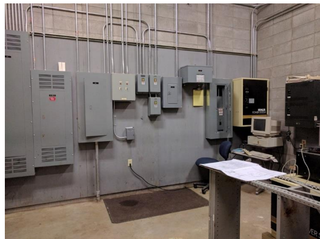
Photo: Panelboards and Transfer Switch
