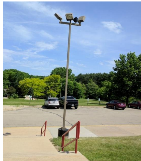
Photo: Exterior Pole Lighting
