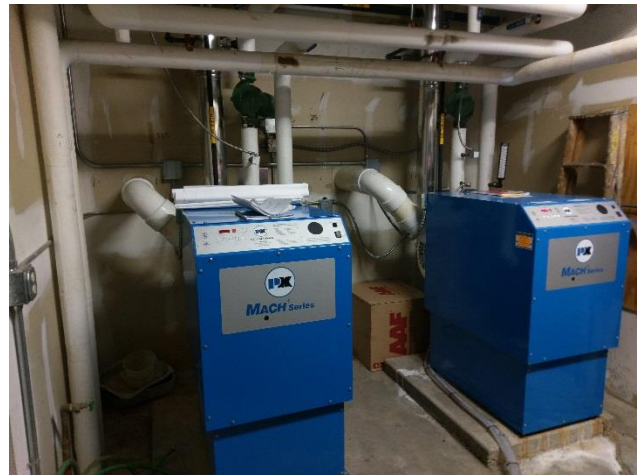
Photo: Hot Water Boilers
