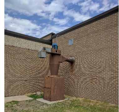
Photo: Dust Collector
