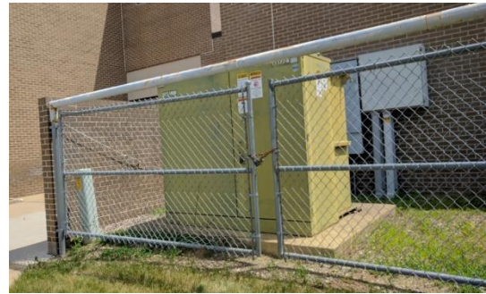
Photo: Alliant Energy Transformer
