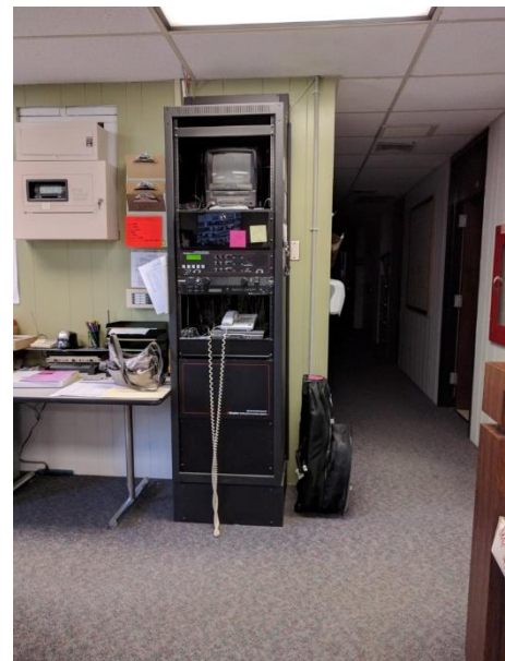
Photo: Public Address System
