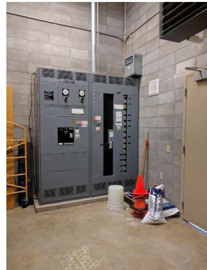
Photo: Main Switchboard
