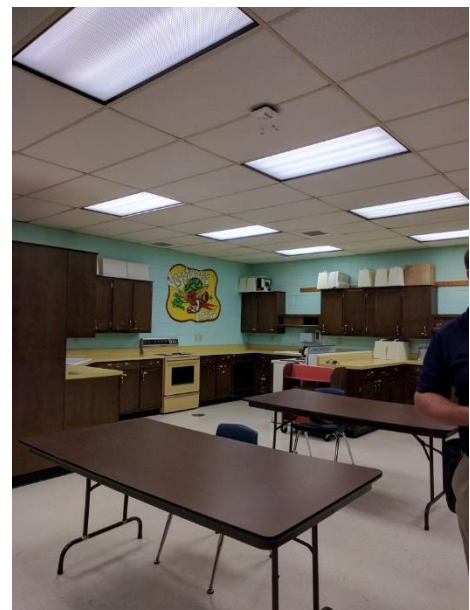
Photo: Typical Classroom Lighting
