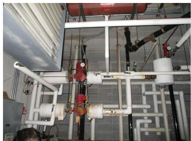
Photo: Hot Water Pumps
