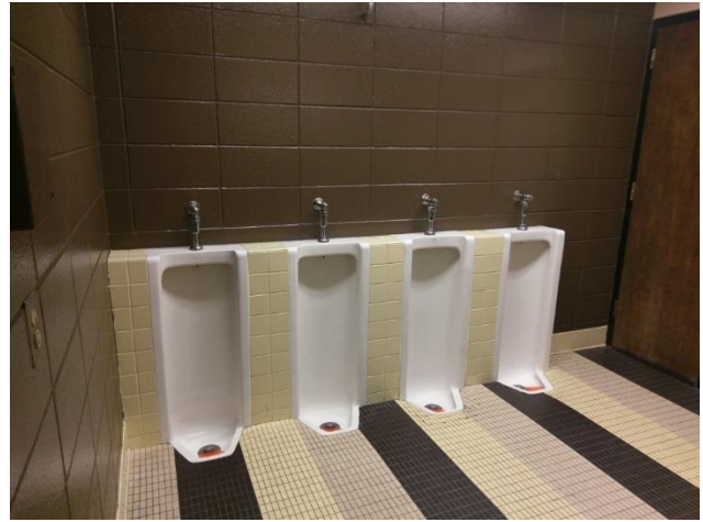
Photo: Restroom Urinals
