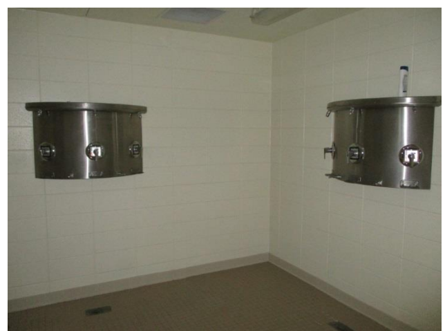
Photo: Shower Fixtures
