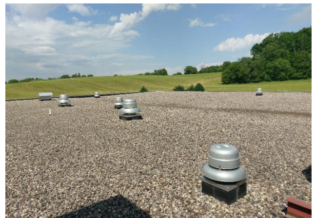
Photo: Powered Roof Exhaust Fans
