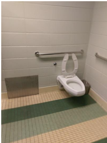
Photo: ADA Water Closet
