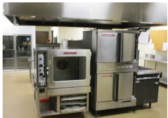
Photo: Kitchen Hood
