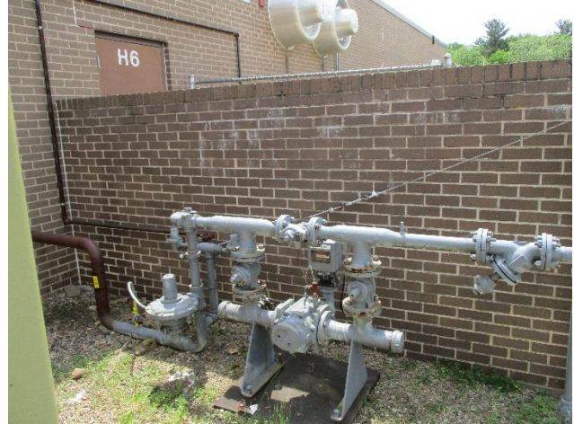
Photo: Main Gas Meter
