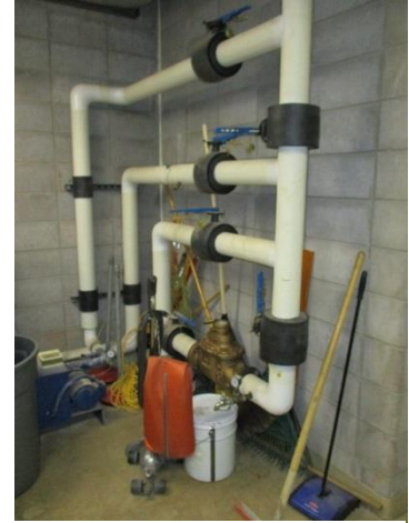
Photo: Main Water Service
