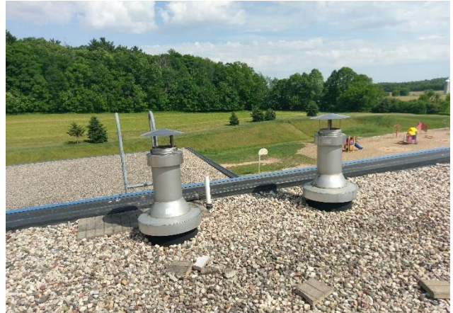
Photo: Existing Boiler's Breeching Stacks
