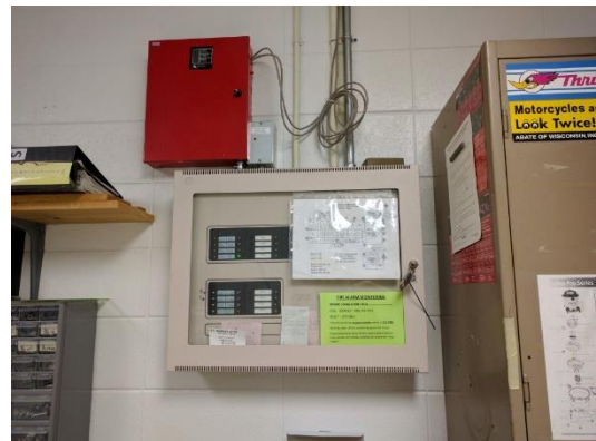
Photo: Fire Alarm Control Panel
