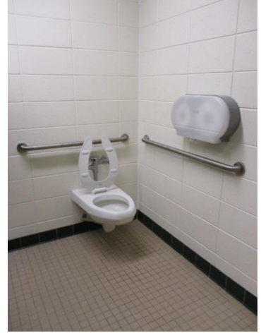
Photo: Wall Mounted Water Closet
