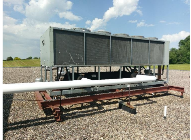
Photo: Air-Cooled Chiller
