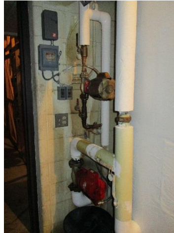
Photo: Recirculation Pumps
