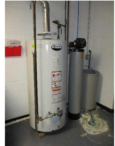
Photo: Kitchen Water Heater
