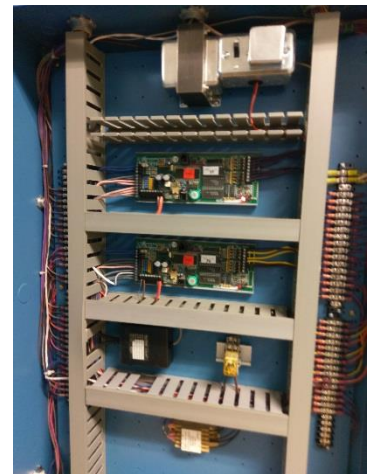
Photo: Direct Digital Controls (DDC)
