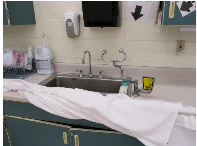
Photo: Art Room Sink - Eye Wash
