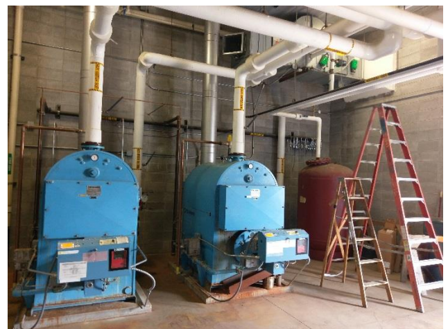
Photo: Hot Water Boilers
