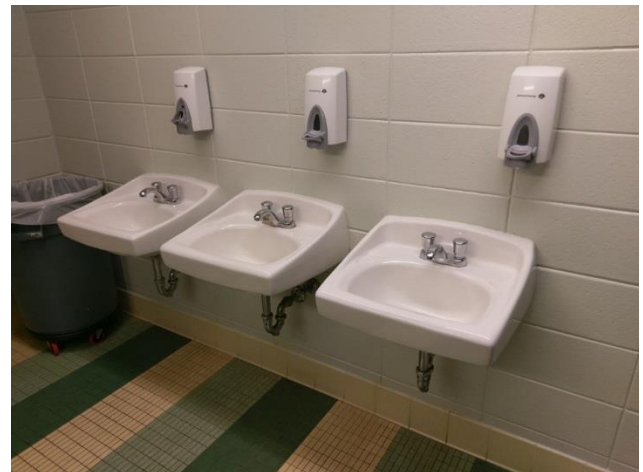
Photo: Lavatory Sinks
