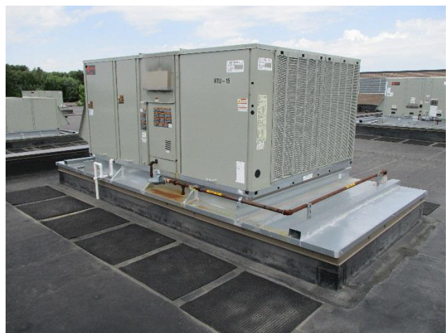
Photo: Gas-fired Rooftop DX Units
