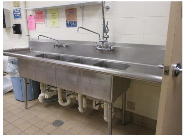
Photo: Four Compartment Sink
