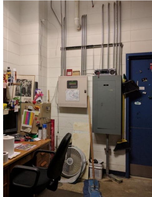
Photo: Fire Alarm Control Panel
