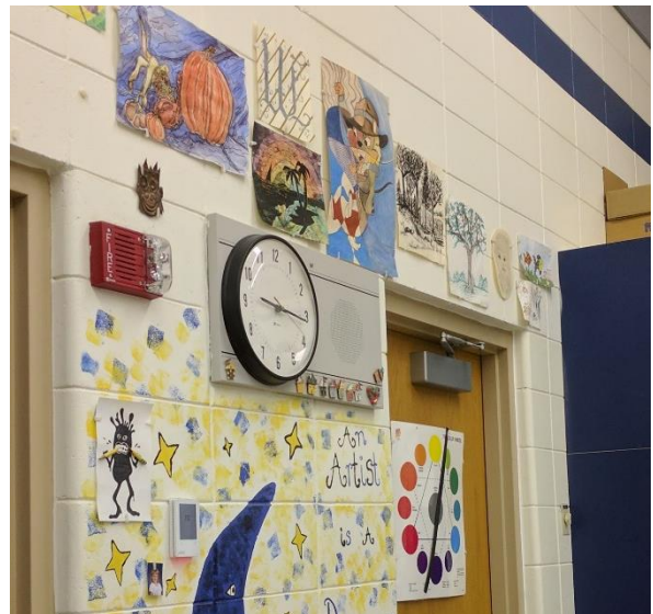
Photo: Typical Classroom Clock/PA
