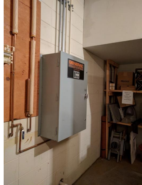
Photo: Automatic Transfer Switch
