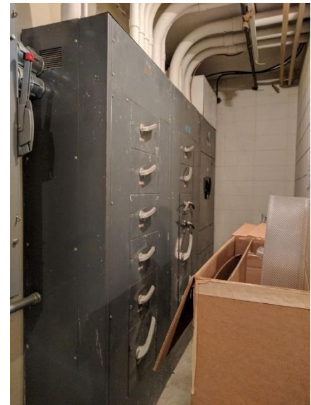
Photo: Main Switchboard
