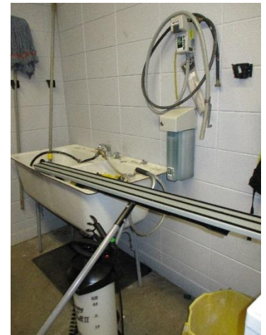
Photo: Laundry Room Sink
