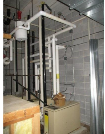
Photo: Hot Water Boilers
