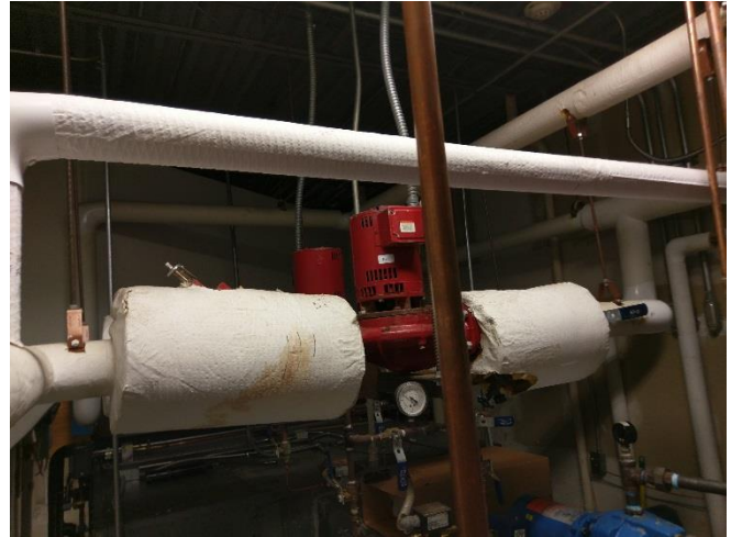
Photo: One Pair of Hot Water Pumps
