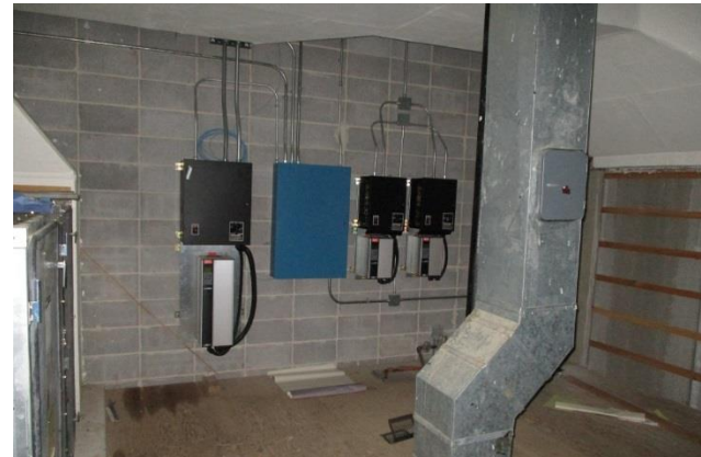
Photo: Direct Digital Controls and VFDs
