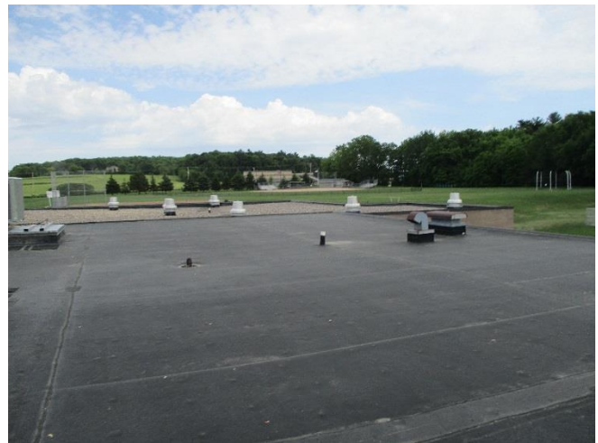
Photo: Power Roof Exhaust Fans
