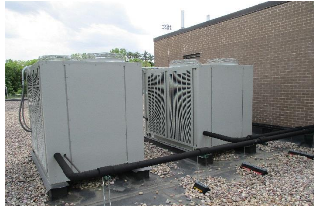
Photo: Air-Cooled Condensing Units
