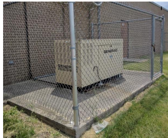
Photo: Exterior Generator
