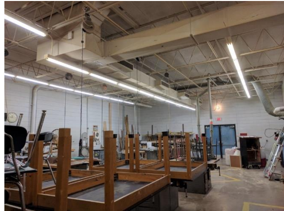
Photo: Typical Shop Area Lighting
