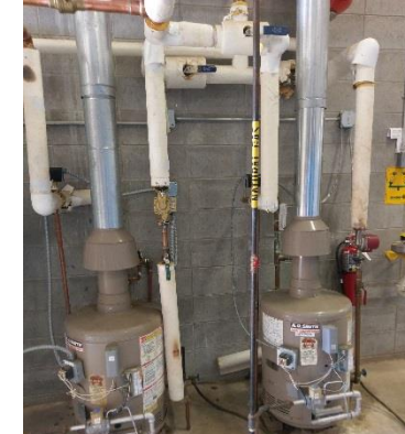
Photo: Main Domestic Water Heaters
