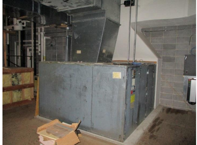
Photo: Indoor AHU
