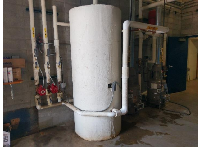
Photo: Storage Tank for Main Water Heaters
