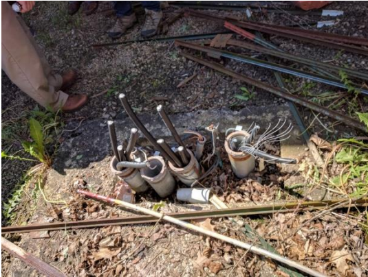
Photo: Old Transformer Location
