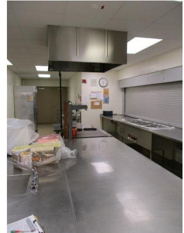
Photo: Grease Hood
